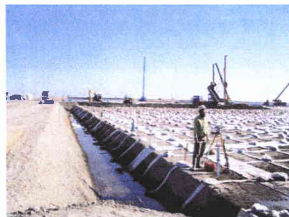
Collecting Ditch in SB Drain System
